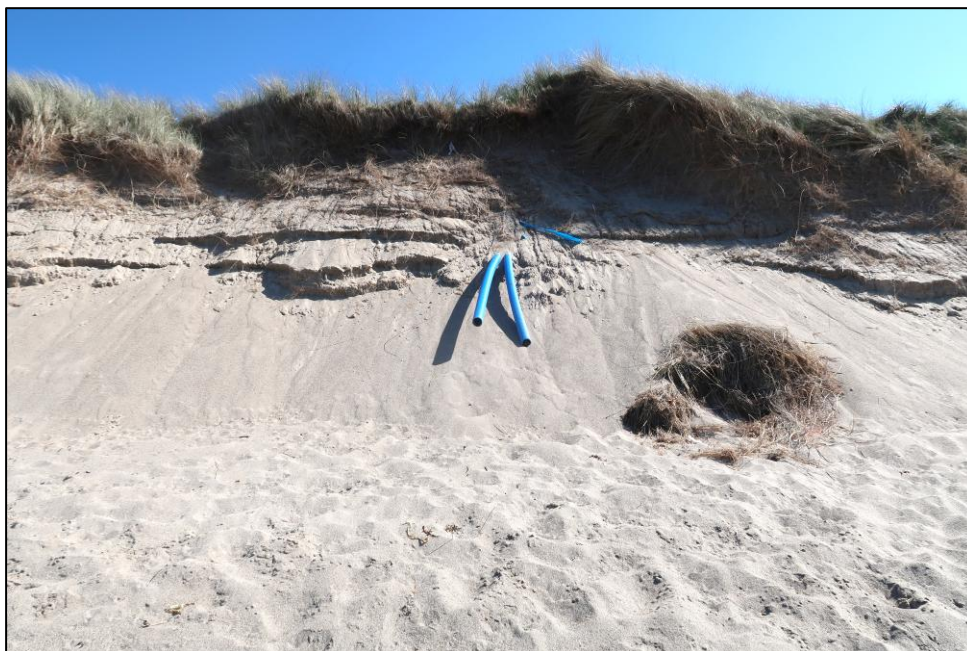
Plate 19. Blue cable ducts and blue tape exposed on the eroding dunes.
